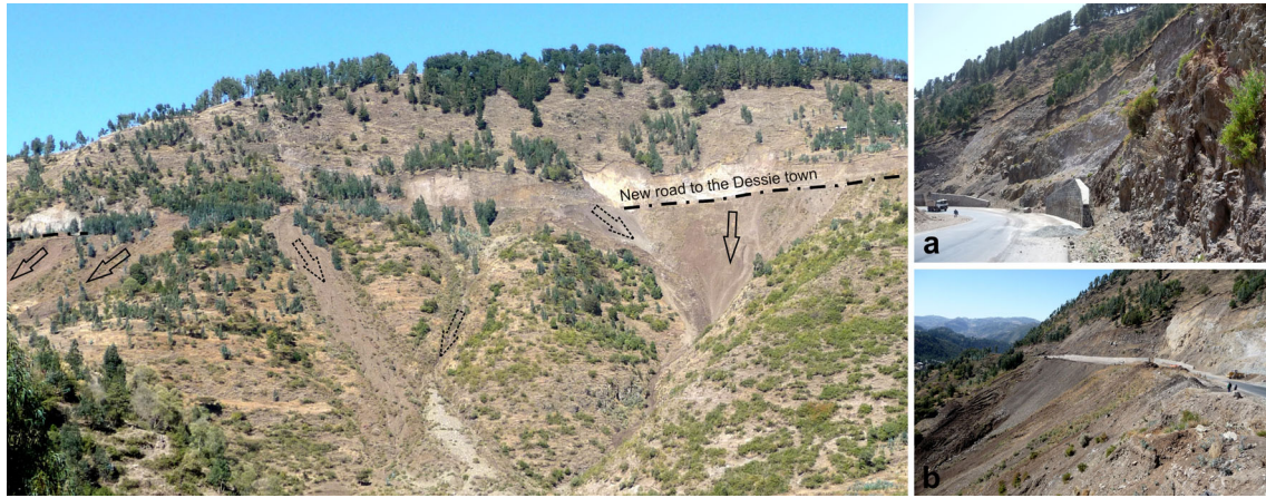
Fig. 6 Several debris flows below the cut of the new road from Kombolcha to Dessie; close-up photos a scarp in stratified volcanic rocks over the road (along with the construction of the massive retaining walls) and b the upper part of the largest debris flow (photo Z. Vařilová)
