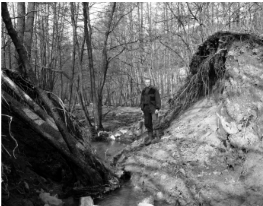
Fig. 3: Detail of the damaged dam of the Blažňov pond
