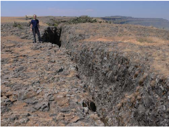
Fig. 1 Opening of tension cracks in the fore field of the upper rim of the plateau above a canyon of nearly 800 m in depth, near Fiche town. Those cracks indicate active, catastrophic rock falls from columnar-jointed tertiary plateau basalts (photo Zvelebil)
