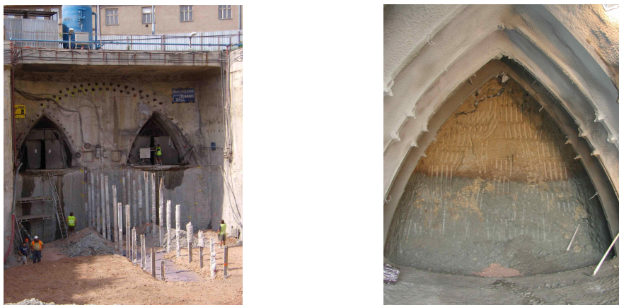
Figure 1: Exploratory adits situated in the tunnel top heading and detail of the left drift excavation
